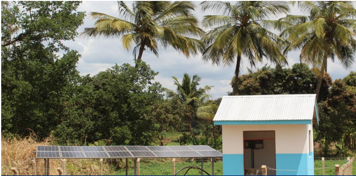
Solar water pumping system constructed by the Water Resources Integration Development Initiative (WARIDI) at Maharaka in Morogoro Region.
