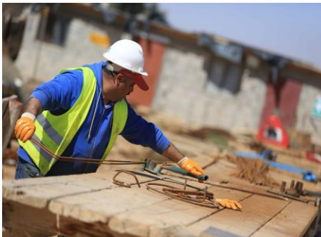
USAID is continuing its 55-year history of partnership with Jordan's government and private sector to build and expand the country's water infrastructure. PHOTO: MOHAMMED MAGHAYDA FOR USAID
