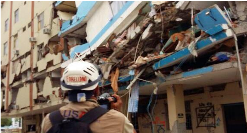
A USAID/OFDA engineering consultant assesses earthquake damage in Manta, Ecuador, in April 2016. Photo by Eddie Argenal/USAID
