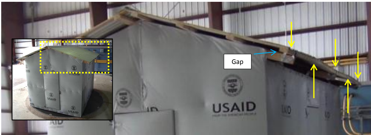
Figure 4 - Windward purlin deformation from uplift forces at 85 mph and 0° angle of attack
