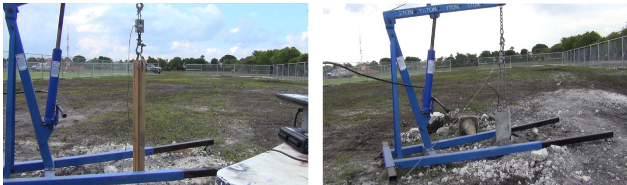
Figure 15 – Pull-out test of footings with hydraulic jack. Left: 4x4 embedded in concrete, right: precast concrete pier
