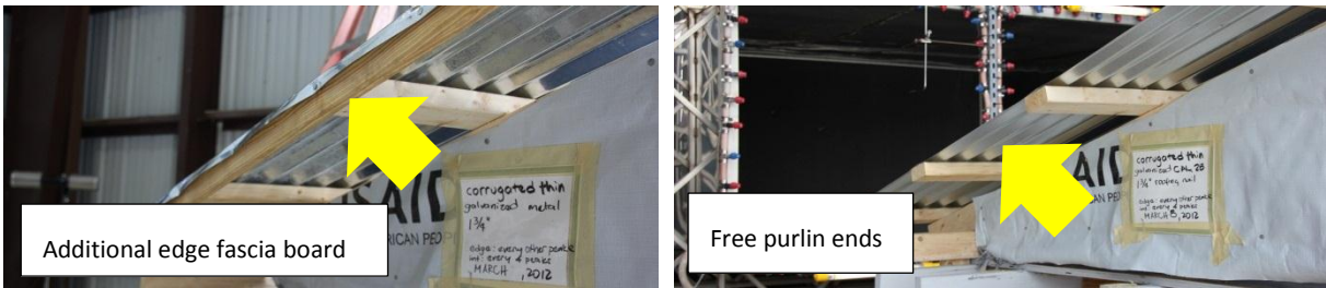
Figure 7 – Roof gable end with additional fascia board and with free purlin ends
