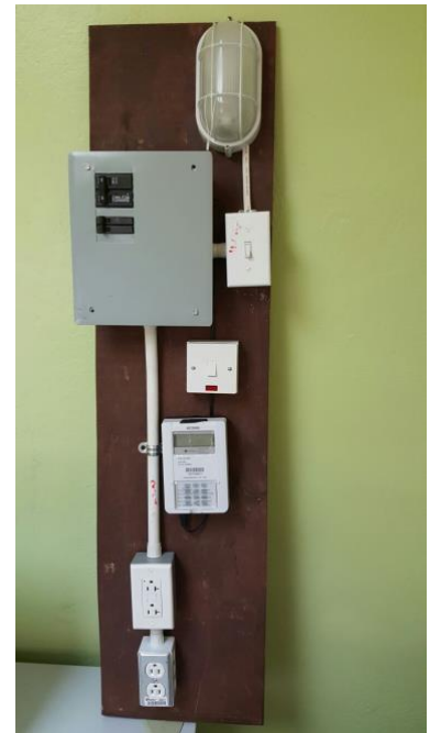
A readyboard customized to the Jamaican electrical and safety standards by JPS engineers.
