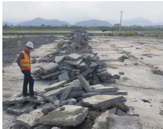
Demolishing the concrete cap of the thermal treatment structure (Photo: CDM Smith)
