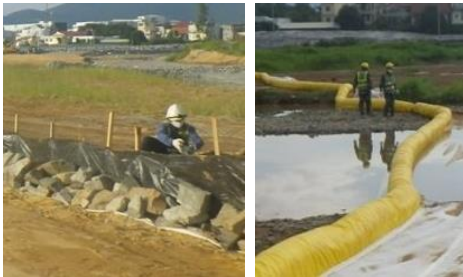
Erosion control measures – silt fences (left) and turbidity barriers (right) (Photos: CDM Smith)
