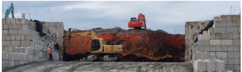
Removing Phase 1 treated soil and sediment from the south wall of the thermal treatment structure (Photo: USAID)
