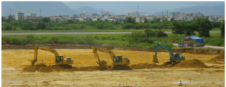
Conducting additional excavation to remove contaminated soil in the Storage Area (Photo: CDM Smith)
