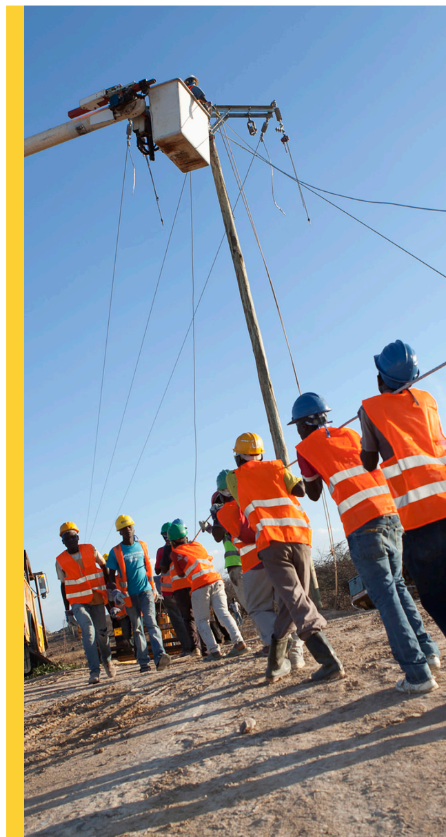
A utility crew from Pike Electric, an American contractor, works to string power lines in rural Dodoma Region, Tanzania. The initiative is part of the Millennium Challenge Corporation's Energy Sector Project. Photo: Jake Lyell for the Millennium Challenge Corporation
