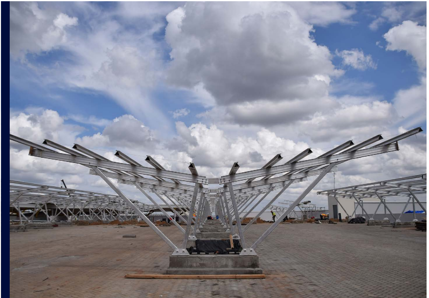
The Garden City solar project site in Nairobi, the largest solar carport in Africa and one of the largest commercial distributed generation sites in sub-Saharan Africa. Photo: CrossBoundary Energy
