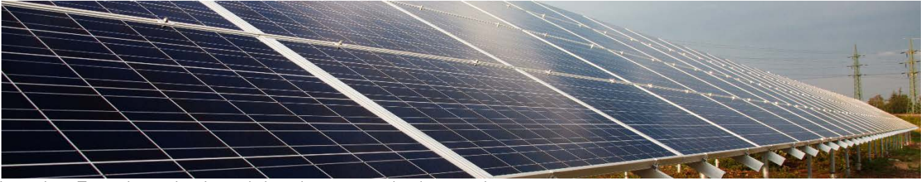
In southern Tanzania, a solar photovoltaic project powers a local community.
