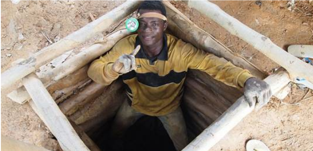
Figure 8. A Ghanaian miner at the opening of a 15-m mine shaft reinforced with wood. Source: https://www.iied.org/ghana-our-way-participatory-reform-artisanal-small-scale-mining-asm-sector .
